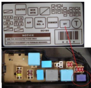
Figure 6 - Example Fuse/Relay Label and Starter Relay Location for a 4.7L Tundra DC – Location/Type May Vary
